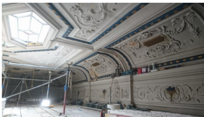
The hole in the ceiling has now been filled by a new plaster panel identical to the one that fell out. Its mould was cast from the facing panel on the opposite side of the skylight which was still intact.
